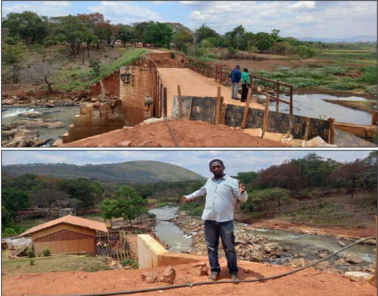
Figure 3: The Chipole Hydro Power Dam after washed by floods
