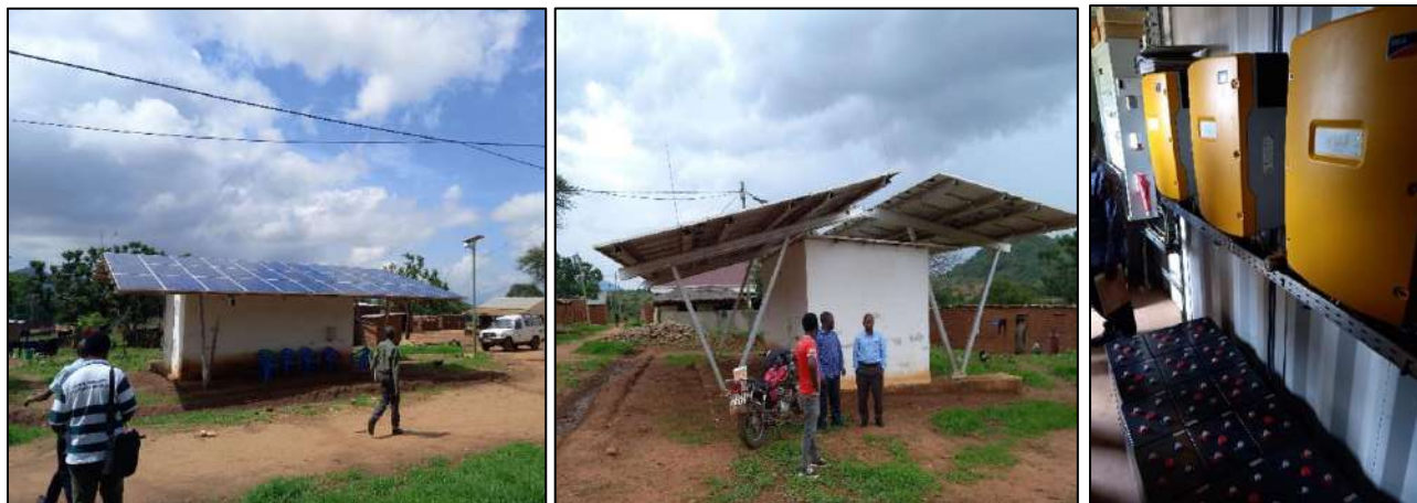
Figure 5: Containerized Leganga Solar PV Mini-grid
