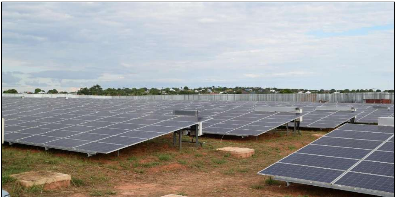
Figure 13: NextGen Solar-Wazi 5MW Power Plant in Kigoma
