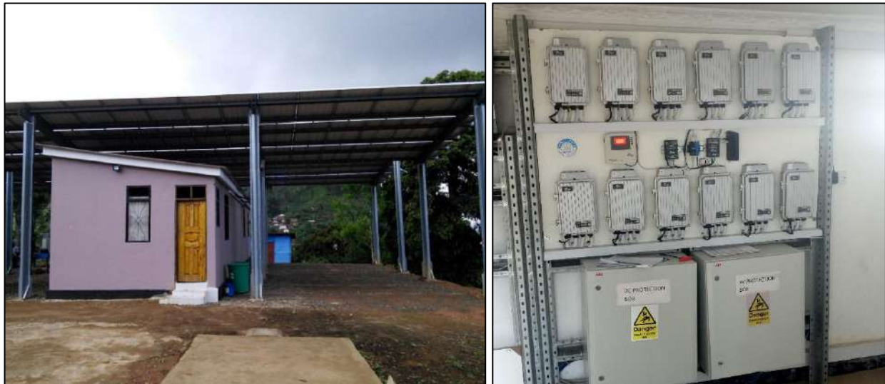
Figure 14: Part of the 48kW Solar PV Mini-grid at Mpale Village, Korogwe, Tanga Region
