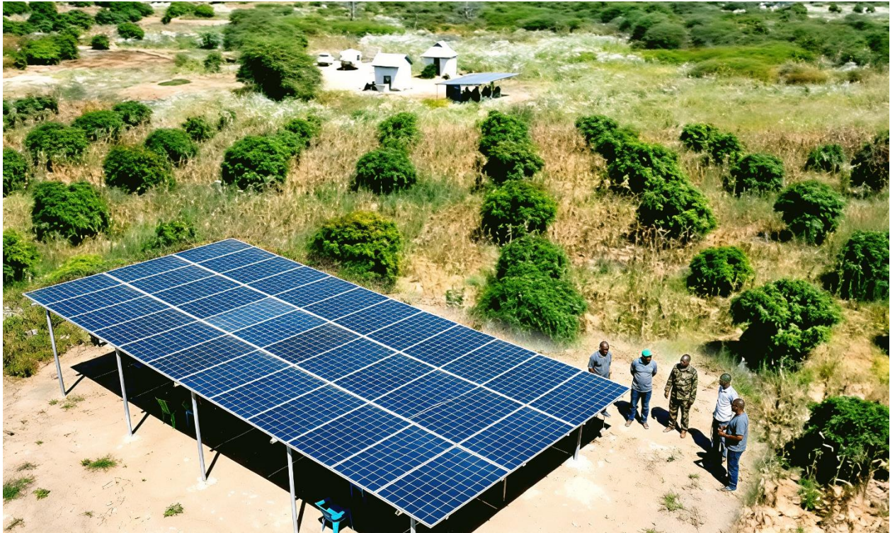
Huzi Drip Irrigation Mango Farm in Chamwino, Dodoma powered with Solar PV system
